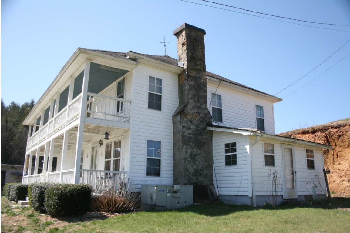
Hickey House, northeast elevation showing new siding and windows, view to southwest
