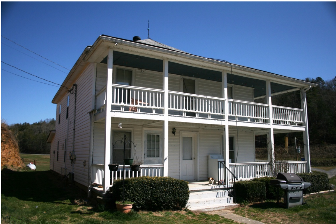
Hickey House, oblique rear view to northeast. New siding on rear elevation and original weatherboards under the porch
